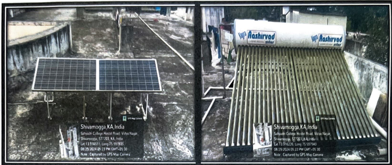
Solar Panels and Solar Water Heater installed at Hostel
